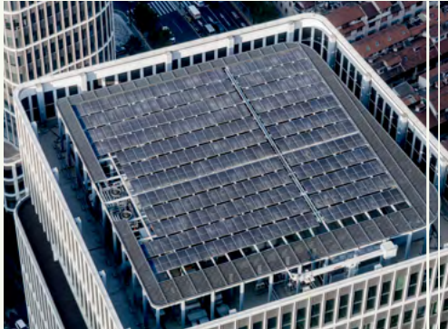
Solar PV panels installed on the roof of CXCC Tower 2
